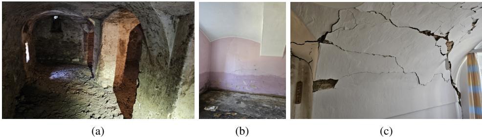
Fig. 4. Nowy Swietow, 22 September 2024: a), b) wet and contaminated floors and walls of basements and ground floors; c) damaged structure of a building dating from the mid-19th century – photo by D. Bajno
