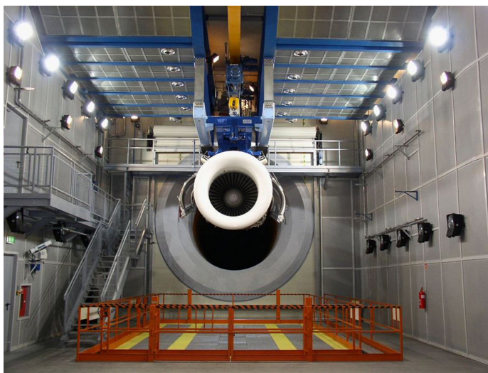
Fig. 3. Engine test stand facility
