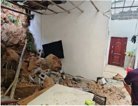
Fig. 5. Landslide site in Xianqiao Village, Lukou Township, Xiushui County, Jiujiang City, June 2024
