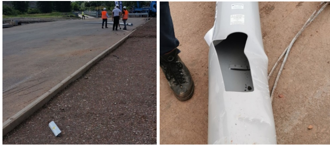
Fig. 11. View of the site of the fallen inspection door and the damage to the column shaft caused when it was pulled out of the ground (source: [33])
