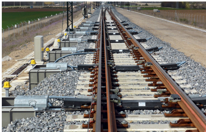
Fig. 4. Turnout type 60E1-17.000/7.300-1:50 on a railway HS line in Spain
