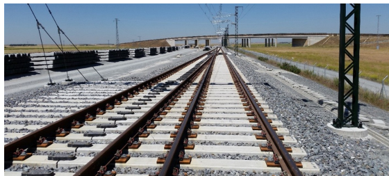
Fig. 1. Turnout type 60E1-17.000/7.300-1:50 on a railway HS line in Spain
