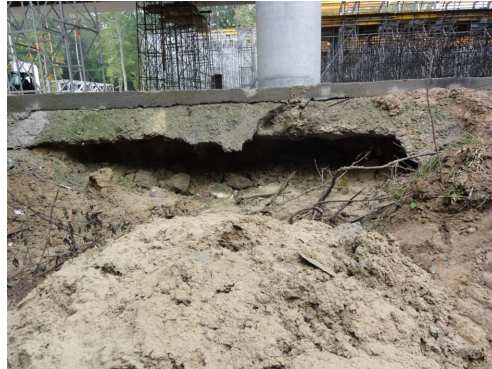
Fig. 8. Voids under the working platform near one of the supports
