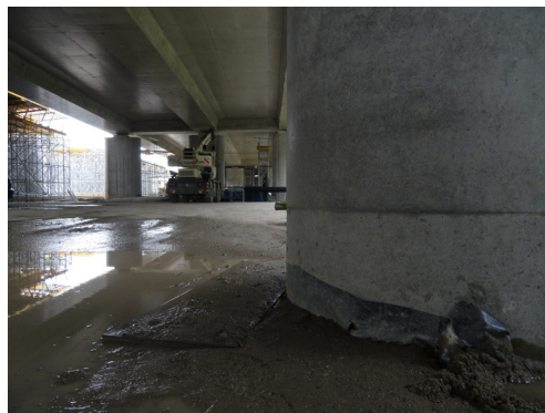
Fig. 7. Deformation and local depression of the working platform near one of the supports
