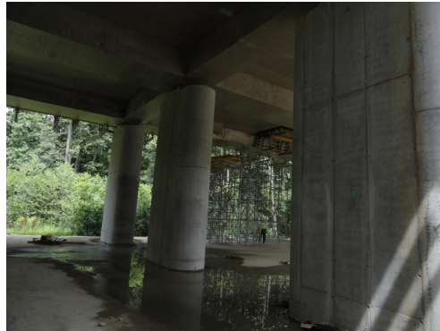
Fig. 6. General view of the oval columns of one of the supports of the left-hand carriageway of the site under consideration
