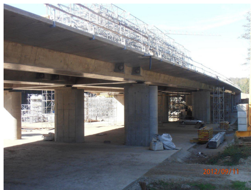
Fig. 5. General view from below of the built superstructure of the left-hand carriageway and the pillars
