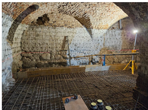
Fig. 2. Construction of a reinforced concrete floor slab and waterproof insulation of walls
