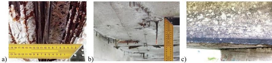
Fig. 8. Bridge corrosion a) prestressing tendon rods view b) stalactites of calcium salt infiltrations c) ASR effect on concrete.
